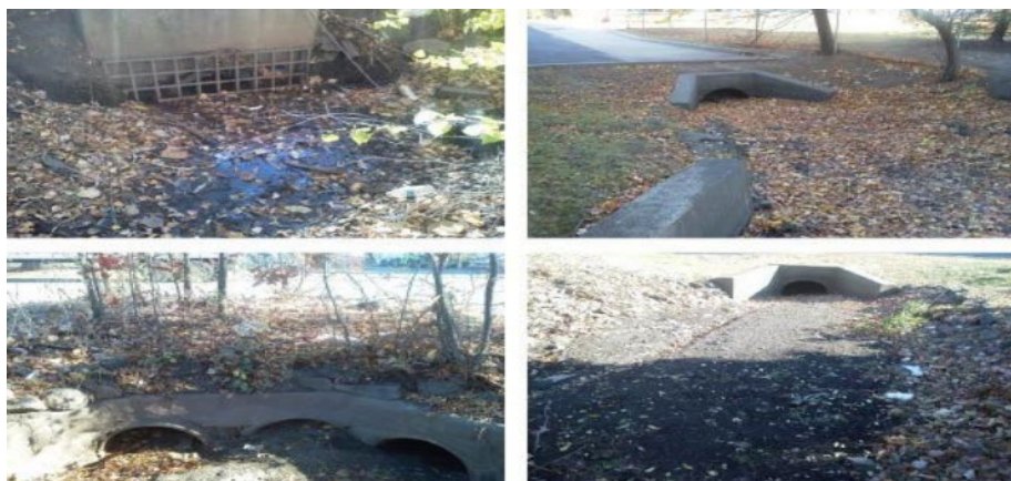
Figure 4-2: Drainage Systems, Moonachie/ Little Ferry. Addressing drainage issues could offer low-cost investment opportunities to increase New Jersey’s flood resilience. For example, bottlenecks in drainage systems, accumulated debris, and overgrowth may collectively exacerbate the impact of flooding and storm surge on communities. In addition, some drainage systems, constructed piecemeal over the last two centuries, have never been mapped. For example, Rutgers has been evaluating how minor drainage improvements can reduce flooding in the Moonachie/ Little Ferry region (pictured).
