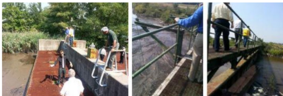
Figure 4-1: Physical Inspection of Existing Risk Reduction Infrastructure. Teams assigned by the New Jersey Department of Environmental Protection have endeavored to catalogue Superstorm Sandy’s impact on berms, tidal gates, and other existing risk-reduction infrastructure. Physical inspection is a key part of the State’s assessment of the current condition of measures to identify necessary repairs as well as opportunities to enhance existing measures to address future extreme weather events and maximize federal investment.
